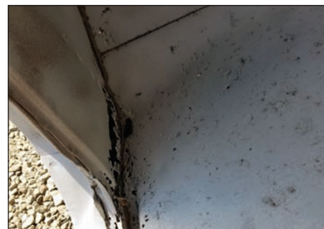
See the rust here and those little pits? Those are some small to large amounts of rust that the media blasting process removed that will need to be replaced. (Photo Courtesy Lonnie Thompson)
