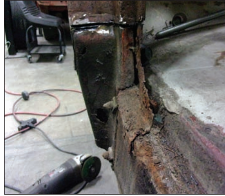
The rockers are always an obvious problem (this goes for most projects, regardless of make), but once you cut away the outer panel, you can see the real problem: the inner rockers. If the outers are gone, the inners probably are too. (Photo Courtesy Lonnie Thompson)
