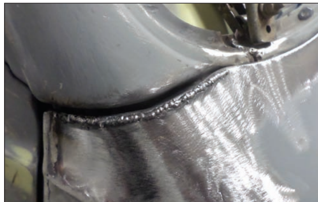
The top part of the cowl by the pillars needed help too. To close that gap, they first cut the cowl with a cut-off wheel and lifted the remaining metal up. Then they filled in that gap with weld as shown. (Photo Courtesy Lonnie Thompson)
