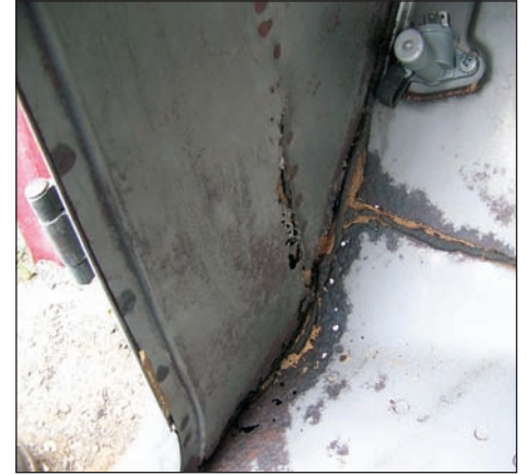
The inner kick panels usually see rust too. In this case, it's not that bad and can be repaired with some home-made patch panels. (Photo Courtesy Lonnie Thompson)
