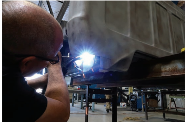
9 Once the piece is cut and shaped, it's tack welded in place inside the cab corner.
