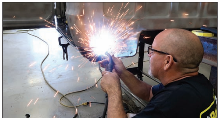
11 The panel is then tack welded in place. Once the panel is confirmed to be straight, he'll finish tack welding the panel and grind down the welds so there's no sign the repair ever happened.
