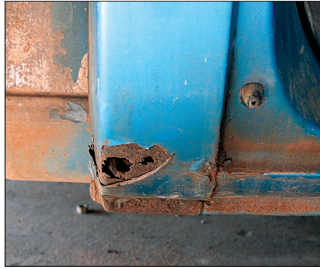
The cab corner on this truck is obviously damaged and needs to be replaced. But how about the rocker just forward of it? In this case, it seemed fine, but it's always good to look for damage if adjacent panels have issues as well. (Photo Courtesy Jefferson Bryant)
