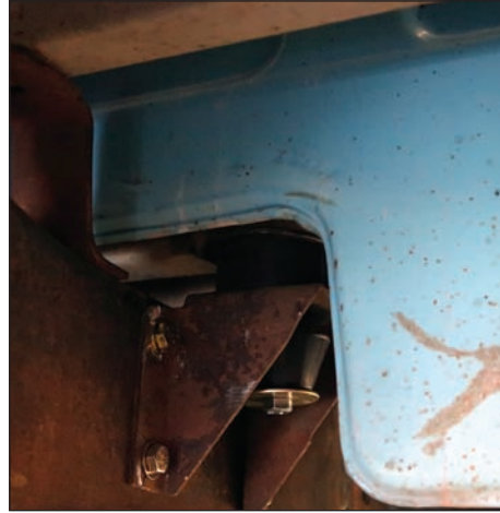
And with both sides in, you can see how the completed setup looks. Now the process just needs to be repeated on the remaining corners.
